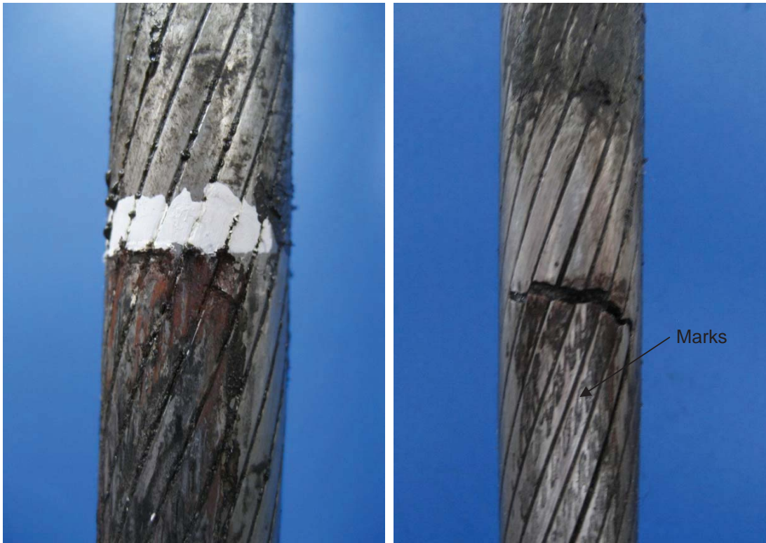
Figure 11: Clamp upper exit point ('front' (left) and 'back' (right)). Note the wire breaks and fretting rounge at the position of the rope just inside the clamp (the edge of the clamp is marked on the front view with the white paint). It is thought that the marks on the Z wires (back view) are from the damage to the clamp from the previous tests on the six-strand rope.
