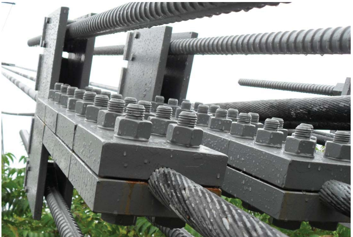
Figure 2: An example of a safety clamp employed on a cable stayed bridge.
